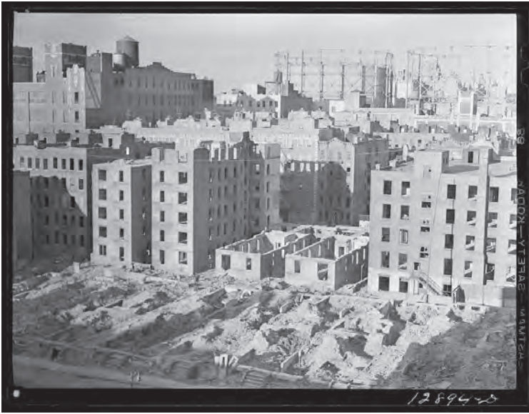
New York, New York. Demolition for slum clearance. Blocks of slum area are torn down for housing project, 1941. Photograph by Edwin Rosskam.
