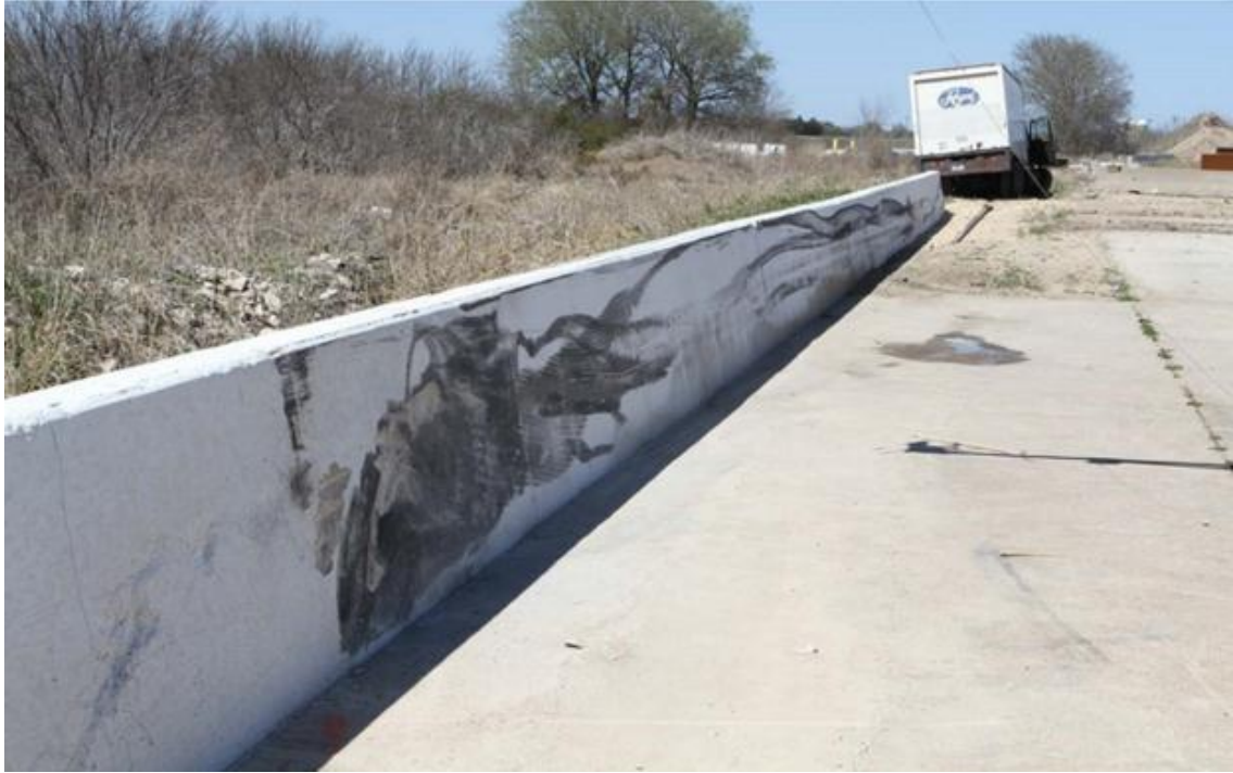
Figure 7: Concrete Barrier Damage after impact – front view (After Sheikh Nauman M., Determination of Minimum Height and Lateral Design Load for Mash Test Level 4 Bridge Rails, 2011)
