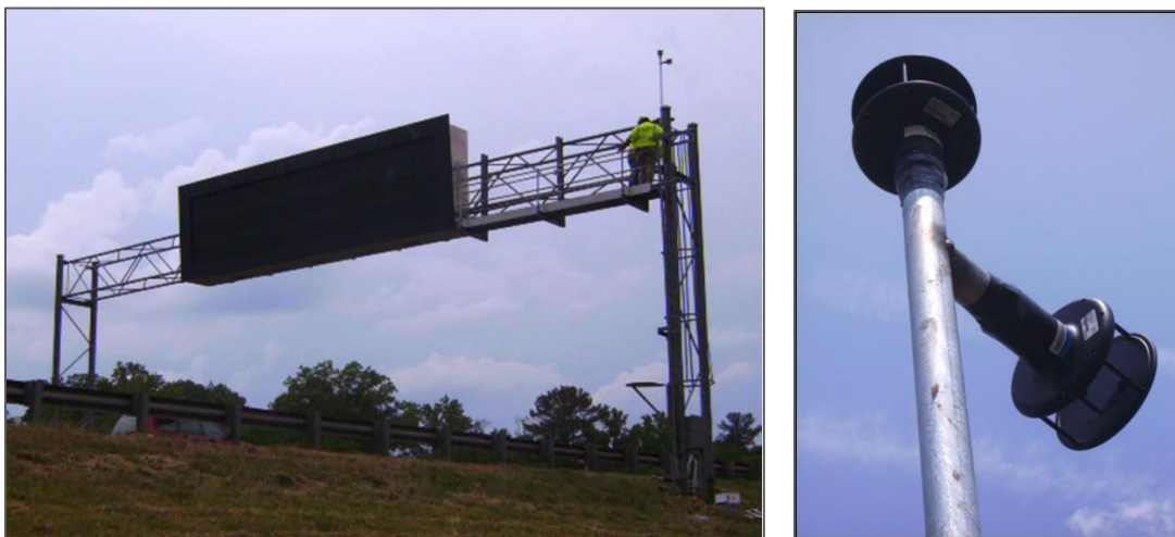
Figure 6-9: Anemometers Connected to Structure with Steel Extension (Fouad 2011)
