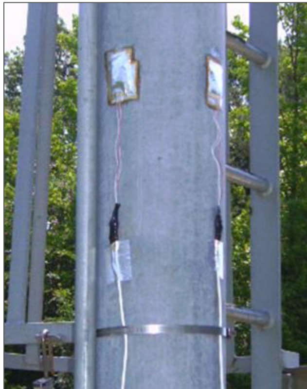
Figure 6-3: Strain Gauges Attached to Upright with Tape at Location 2 (Fouad 2011)
